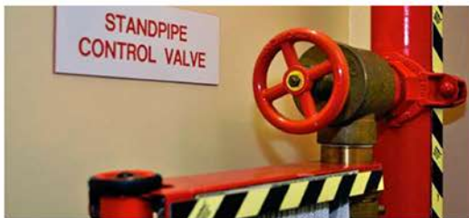
Standpipe Control Valve
